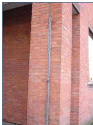
Figure 53. External protection should be provided against damage and vandalism.
